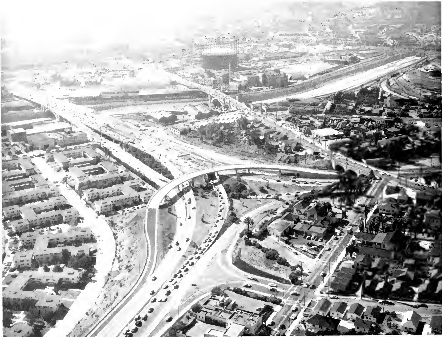
Looking northwesterly toward Santa Ana-San Bernardino interchange with widening construction in progress on Los Angeles River bridge shown center left
